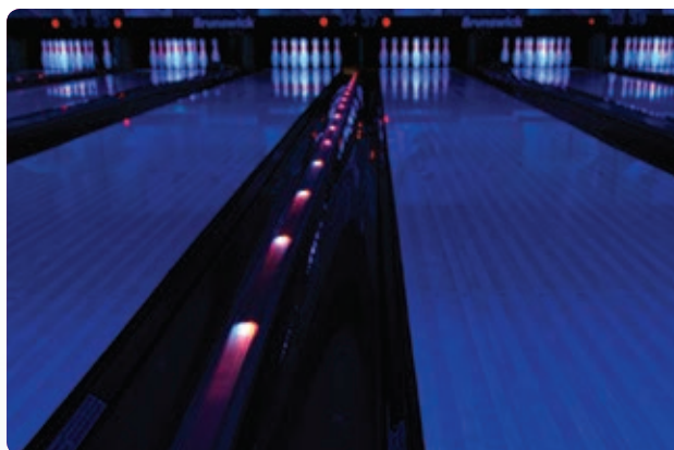
Lightworx Division Lighting System
